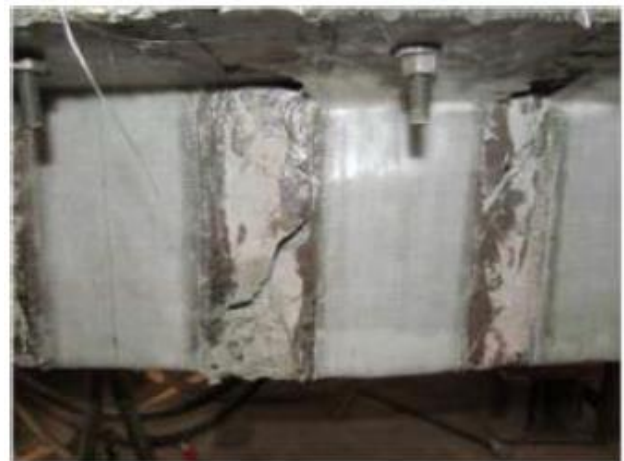
Fig - 1 A View of Crack
